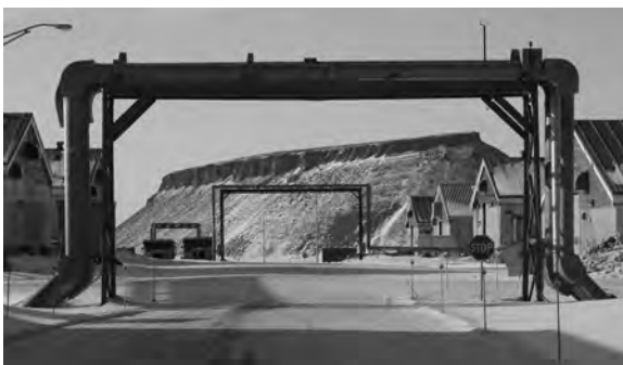
Mount Dundas framed by Thule Air Base's piping system. Credit: Chris Chrissotimos.
